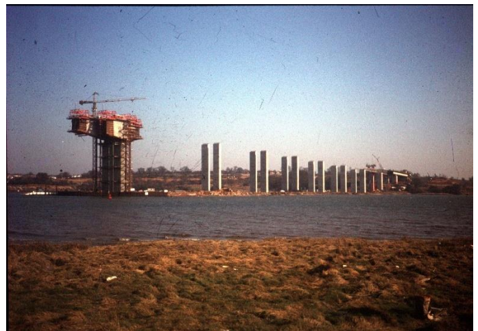
Construction of the Orwell Bridge in the early 1980s. Credit: The Ipswich Society
